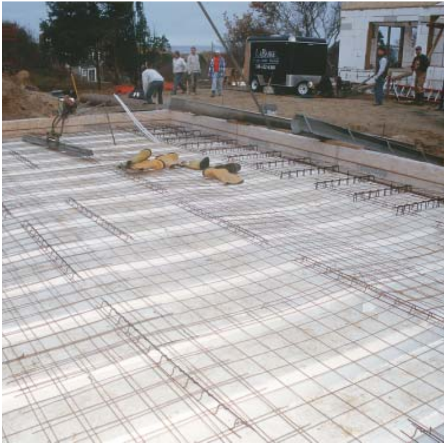
Figure 10. Welded 6-inch-square steel fabric was placed over wire chairs and wire-tied to the perimeter rebar to unify the floor system.
