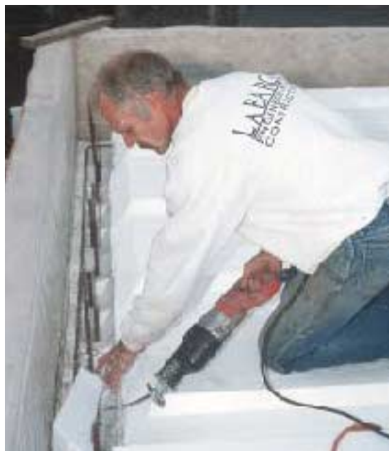
Figure 8. Form edges are eased to reduce the likelihood of a stress crack forming at the transition from horizontal to vertical concrete. The site supervisor approximated the panels' factory longitudinal bevel across the end cuts, using a reciprocating saw.
